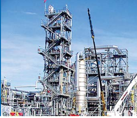
Commercial Geminox® Plant in Lima
